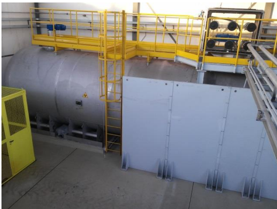
Figure 2: View of tank with shielding wall covering half of side of the tank
